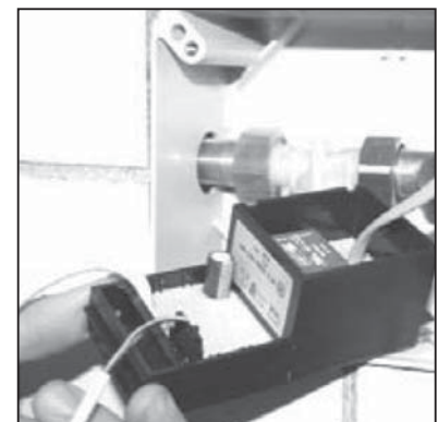
Connect sensor-siphon to electronic module
